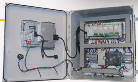
Low Voltage Control Box
